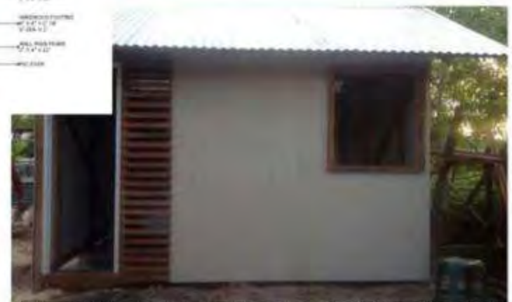
Front elevation of the house. Bottom ready for 1 layer of CHB and concrete floor pouring by owner.
